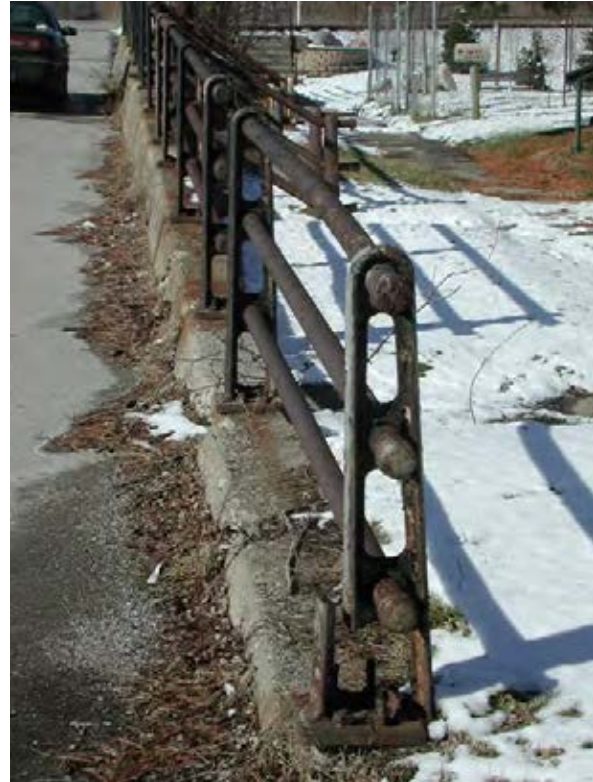
Close-up view of metal railing once used by the railroads. Source: Storrow Kinsella Associates, Inc
